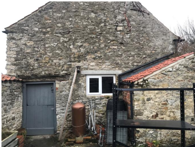
Pic 7 - View onto the eastern façade. Existing historical door, lintel. Later addition of window. New loft access style window in this gable
