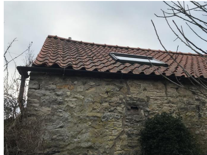
Pic 7 - View looking south onto the northern roof. The existing roof lights are visible at close proximity on the rear
