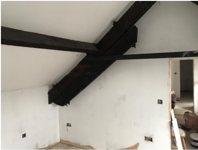
Pic 9 – Internal view of first floor - preserved supporting truss and purlins throughout.
